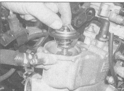
5.7a Lift the thermostat from its housing ...
