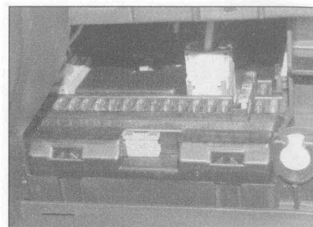
3.3c ... to access the main fusebox
